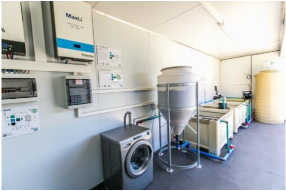
Figure 8: Interior of the LaundReCycle pilot plant including washing machine and installations for the water treatment
