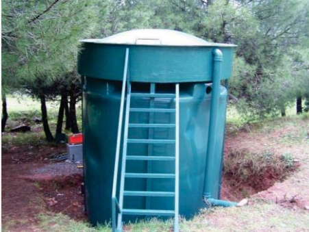
sand-anthracite filter – storage tank
