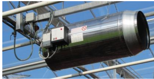
Heating and CO2 supply
