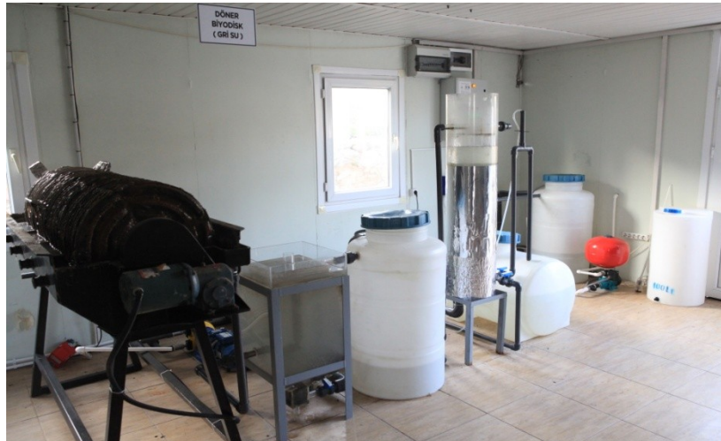
Grey water treatment reuse with RBC- at MRC premises
