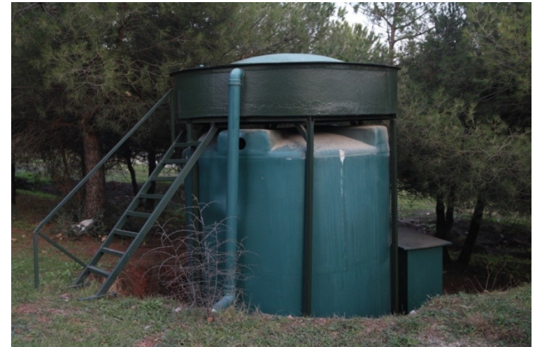
Rain water reuse – anthracite –sand filter, storage
